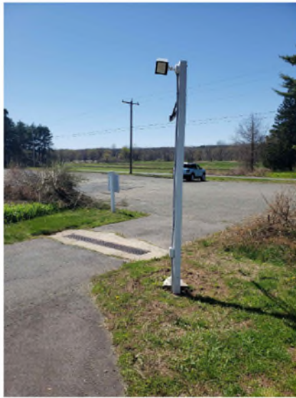
76 EXISTING POLE MOUNTED LIGHT
